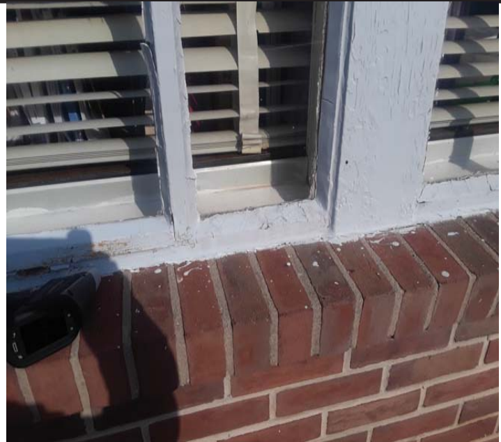
Picture 4: Exterior White Metal Window Casing
