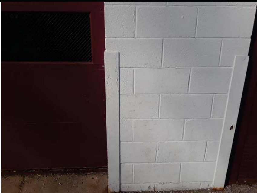
Picture 11: Exterior White Metal Wall Support
