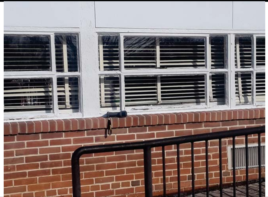
Picture 10: Exterior White Metal Window Casing
