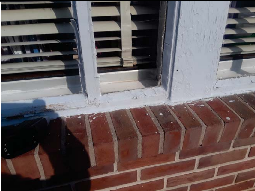
Picture 9: Exterior White Metal Window Casing
