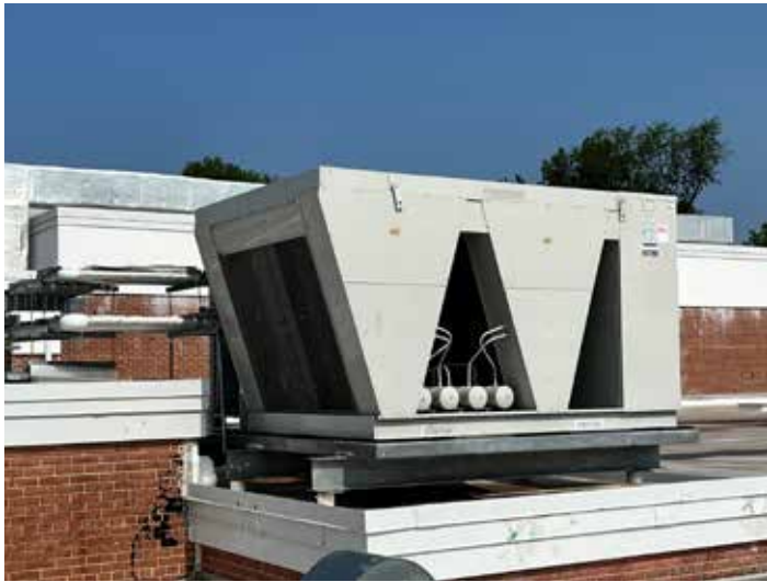
Existing Condensing Unit
