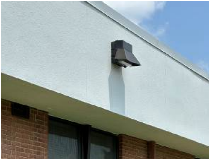
Exterior Canopy Lighting
