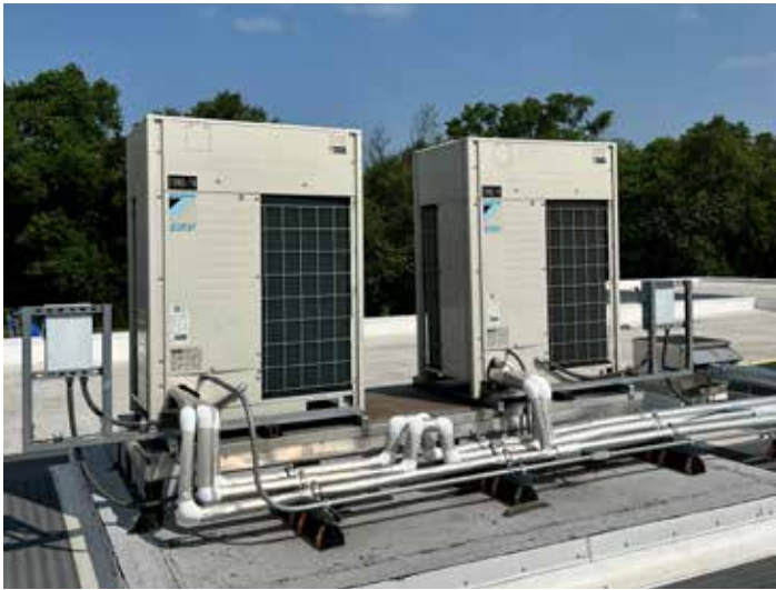
Existing VRF System
