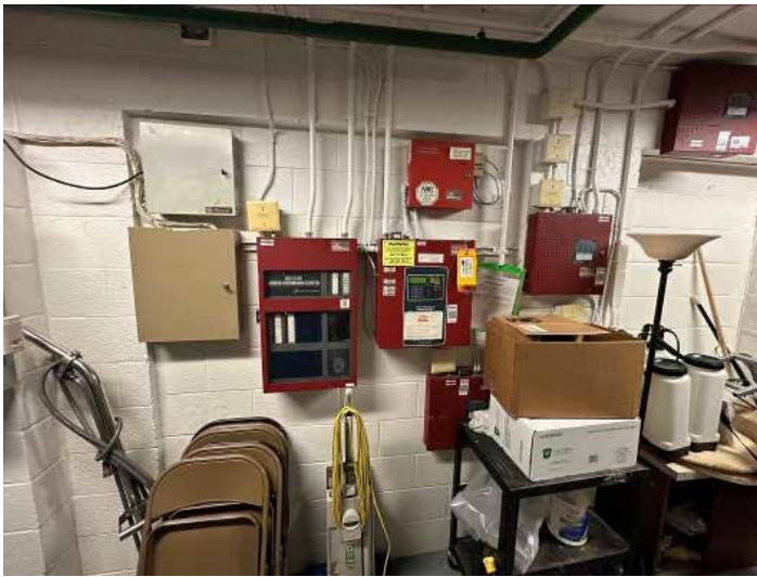
Existing Fire Detection and Alarm Systems
