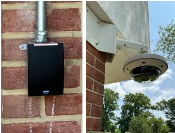
Exterior Card Reader and Video Surveillance Cameras
