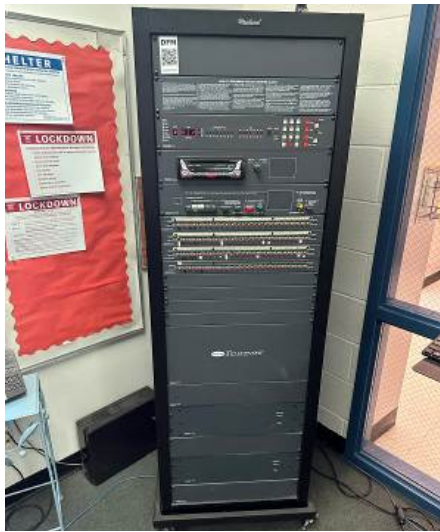
Intercom Main Console
