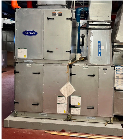
Existing Air-Handling Unit (AHU-6)
