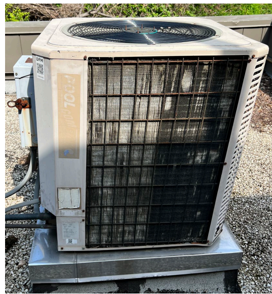
Existing Air-Cooled Condensing Unit
