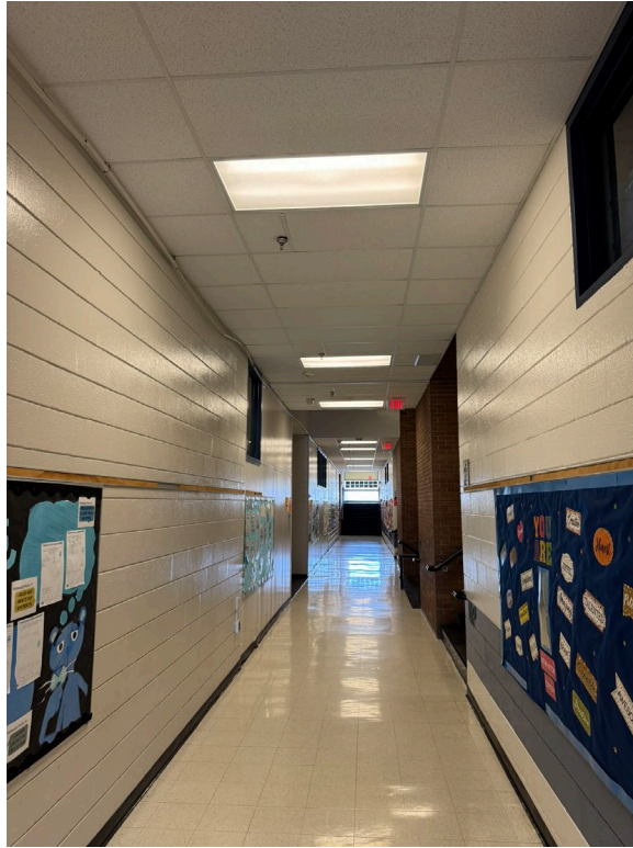
Typical Corridor Lighting
