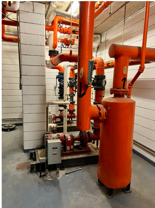
Existing Heating Water Pumps and Air Separator
