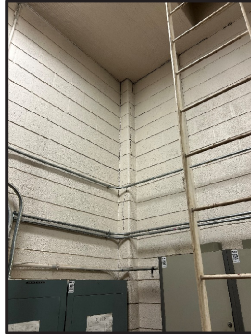
Figure 4 Mechanical penthouse wall cracking.
