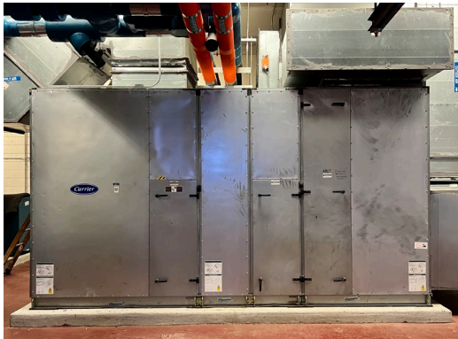
Existing Air-Handling Unit (AHU-7)
