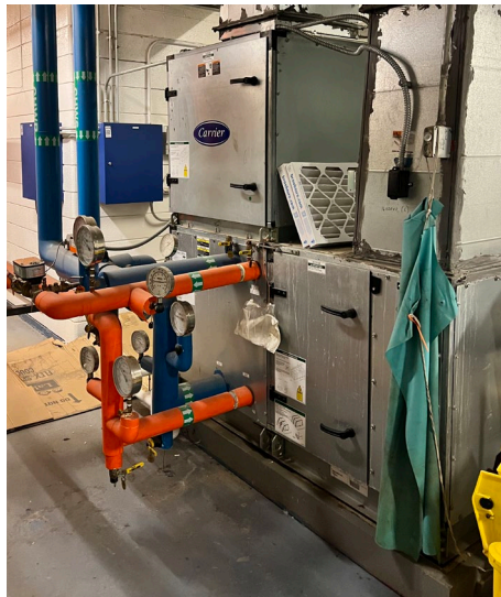
Existing Air-Handling Unit (AHU-2)
