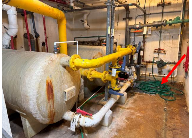
Photo #16 View of pool filters and backwash tank.
