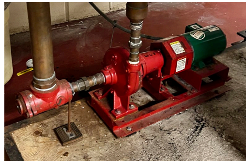
Existing Pool Circulator Pump
