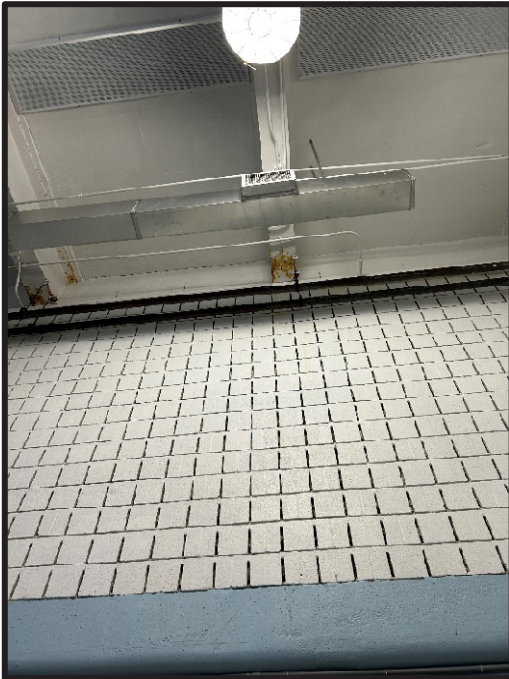
Figure 1 Beams at bearing location in pool area showing corrosion.
