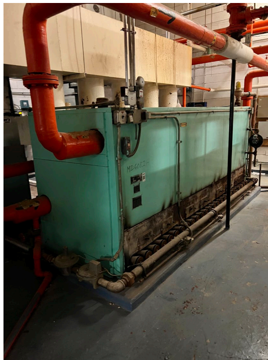
Existing Hydronic Boilers
