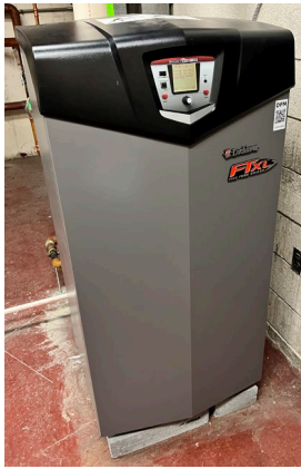
Existing Pool Boiler
