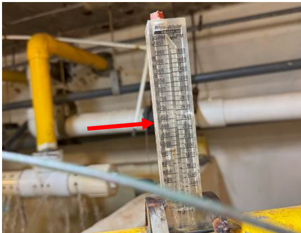
Photo #21 View of pool flow meter reading 425-gpm.
