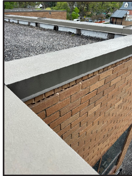
Figure 6 Displaced brick at top of parapet.
