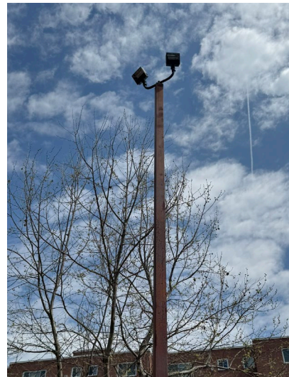
Exterior Pole Mounted Lighting Fixture
