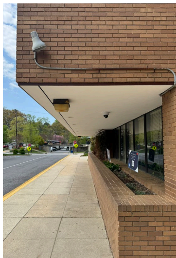
Exterior Lighting Fixtures
