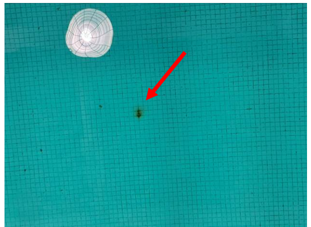
Photo #6 View corrosion stain at pool floor tile.
