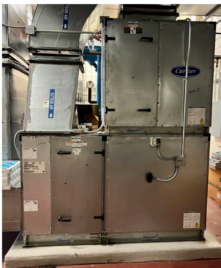
Existing Air-Handling Unit (AHU-5)
