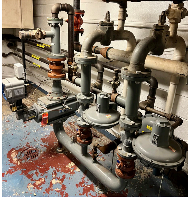
Existing Gas Service and Washington Gas Meter
