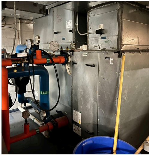
Existing Air-Handling Unit (AHU-1)
