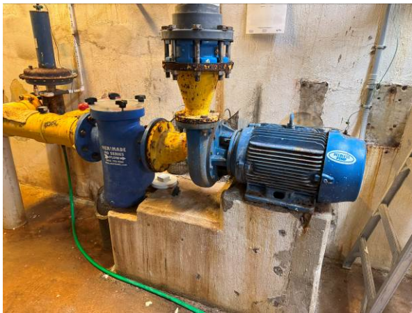
Photo #15 View of pool pump, piping and valves.
