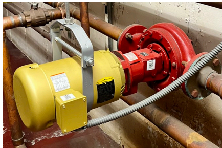
Existing Boiler Circulator Pump
