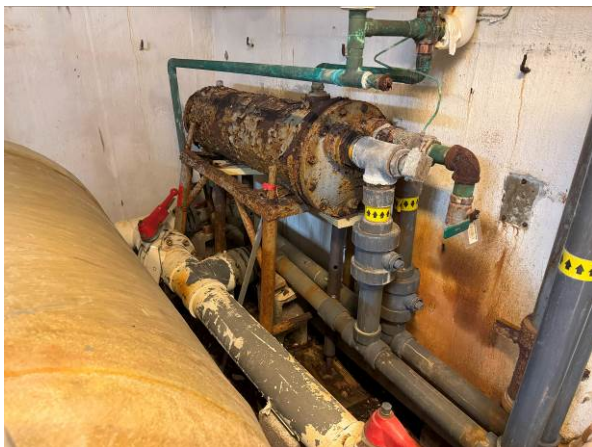
Photo #17 View of pool heat exchanger and piping.
