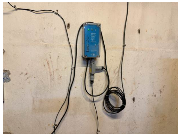
Photo #20 View of pool automated domestic water control panel.
