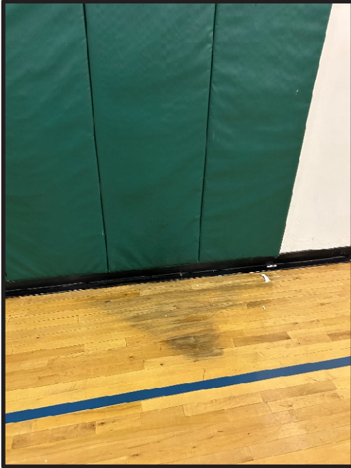
Figure 3 Water intrusion staining in gym floor.
