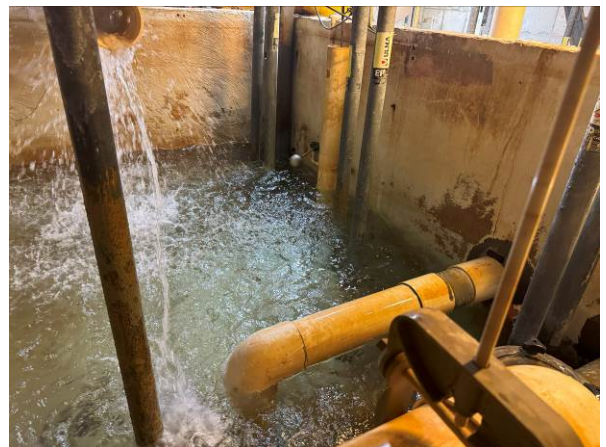
Photo #24 View of pool surge tank suction piping to pump.
