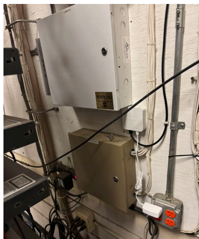
Intrusion Detection System Control Panel
