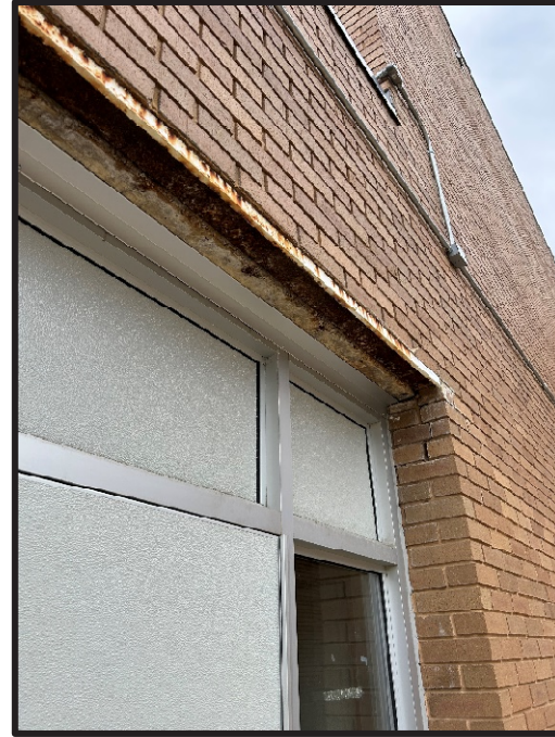
Figure 8 Lintel over window opening showing corrosion.
