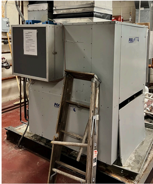
Existing Pool Air-Handling Unit
