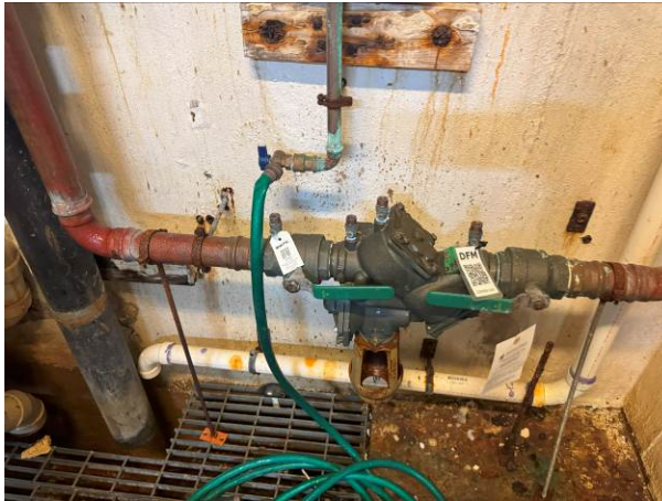
Photo #19 View of domestic water backflow preventer and backwash tank.
