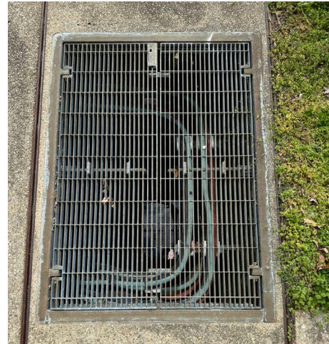
Utility Transformer in Underground Utility Vault
