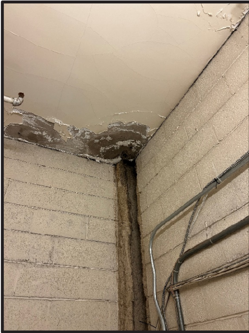
Figure 5 Water intrusion in mechanical penthouse stair ceiling.
