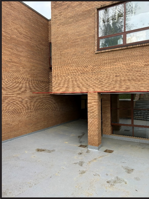
Figure 9 Deflected floor area at rear of building with horizontal reference line.
