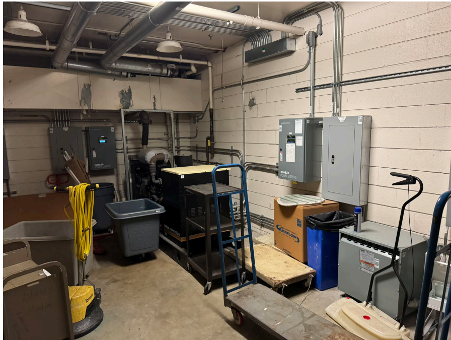
Indoor Generator and Automatic Transfer Switches
