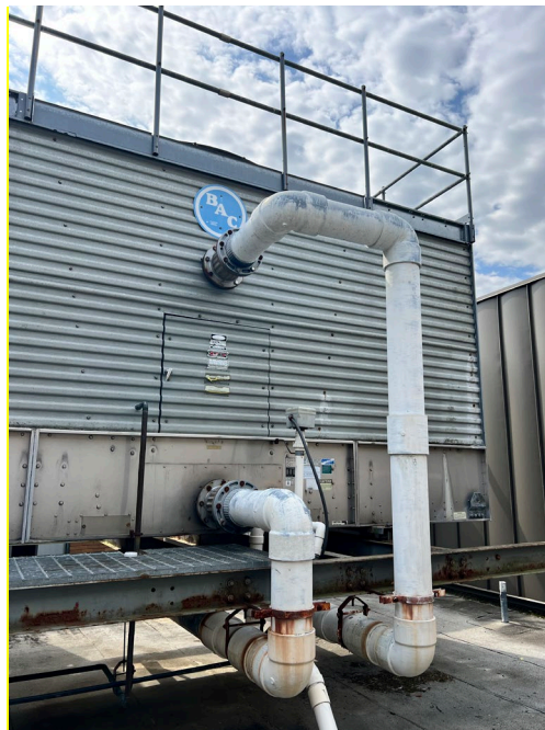
Existing Cooling Tower
