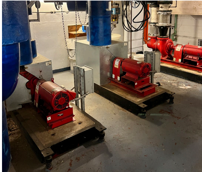
Existing Chilled and Condenser Water Pumps
