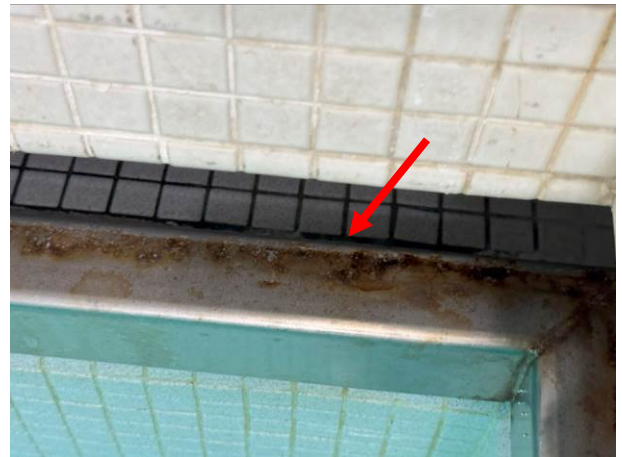
Photo #4 View of pool stainless steel gutter staining and tile finish.
