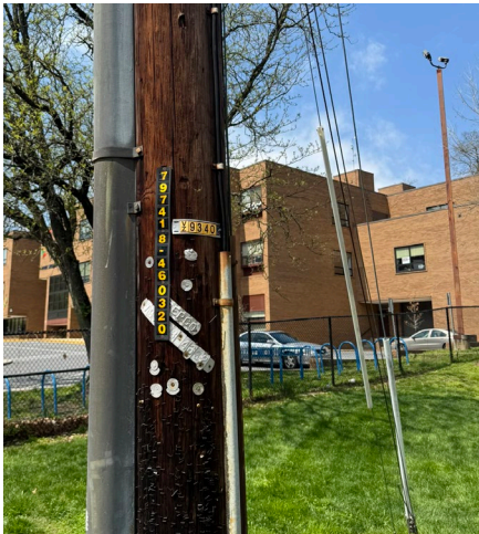
Utility Pole at Maple and Lee
