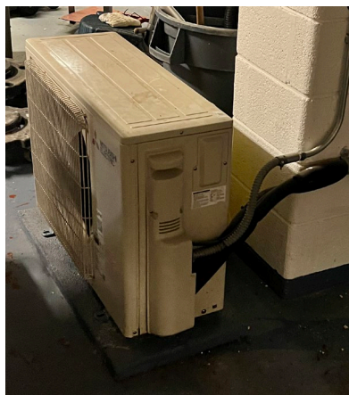
Existing Ductless Split System
