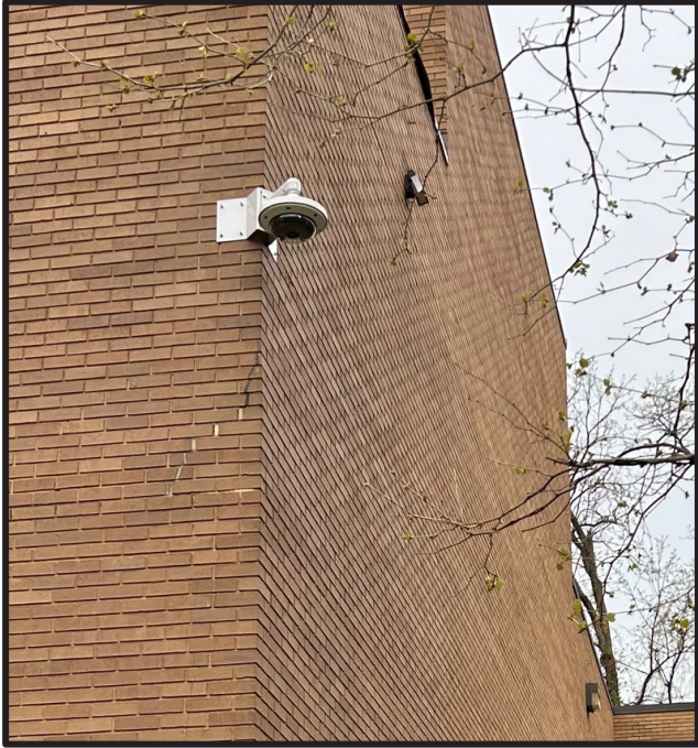
Figure 7 Step cracking at corner of building.
