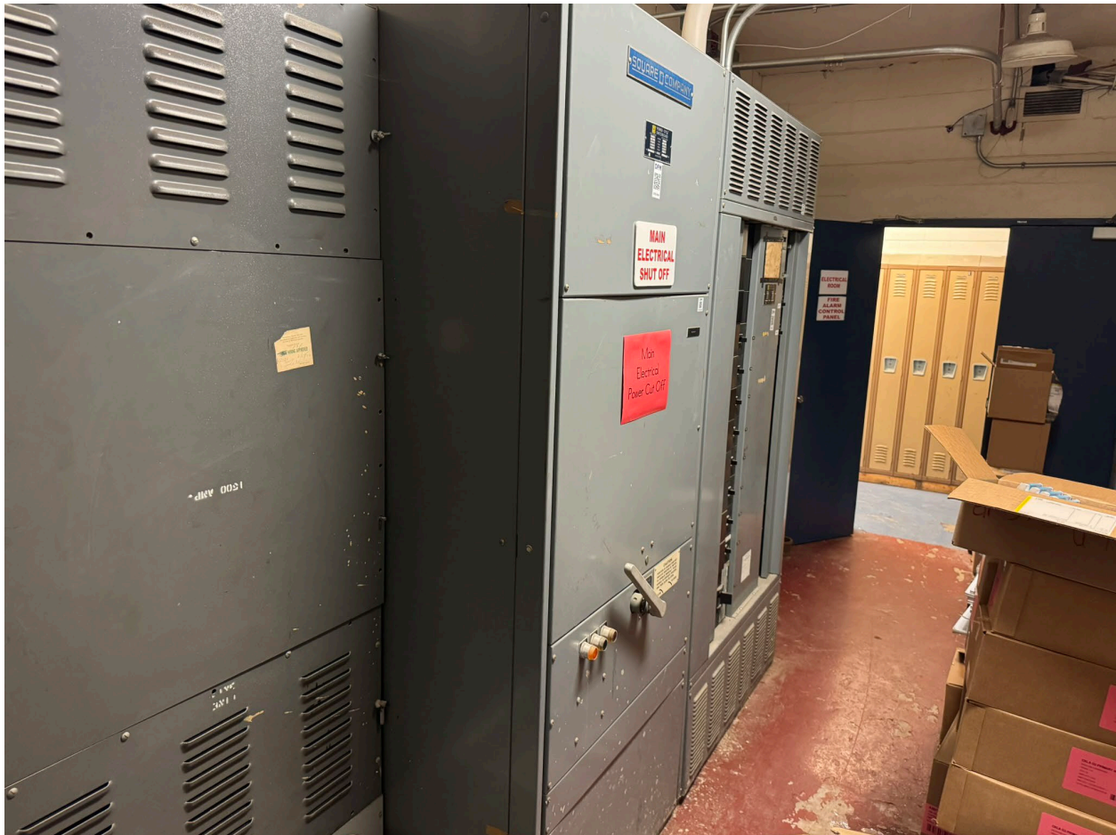
Main Service Switchboard
