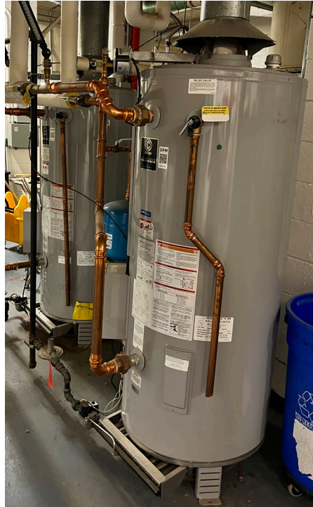
Existing Domestic Water Heaters
