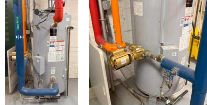
Domestic Water Heater and Domestic Hot Water Circulation Pump
