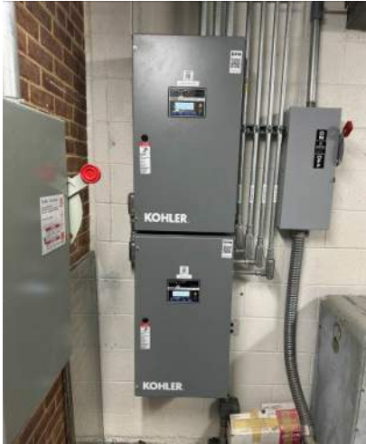
Existing Automatic Transfer Switches
