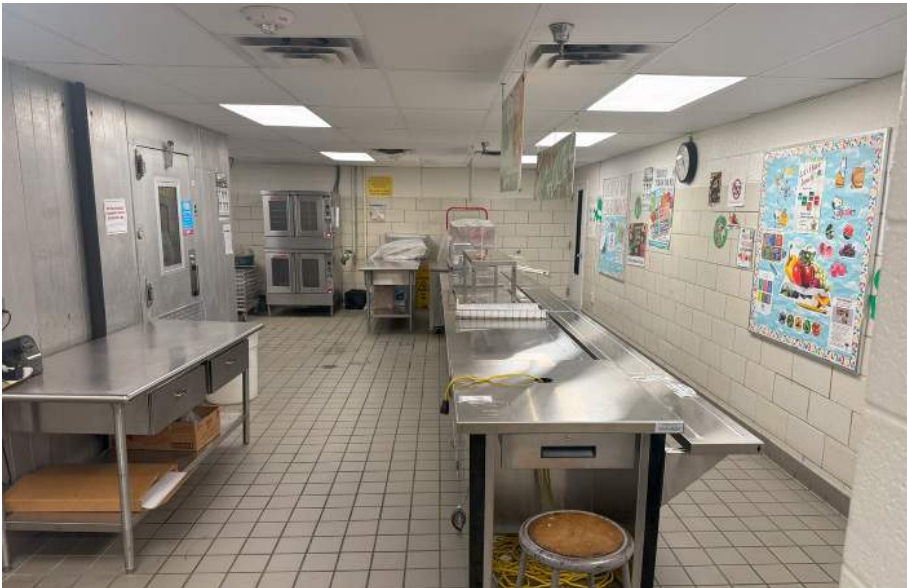
Kitchen Area, Including Overhead Supply Diffusers
