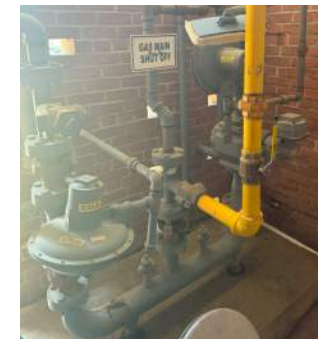
Incoming Natural Gas Service
