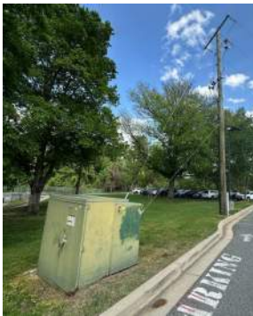
Existing Pepco Utility Transformer and Pole
