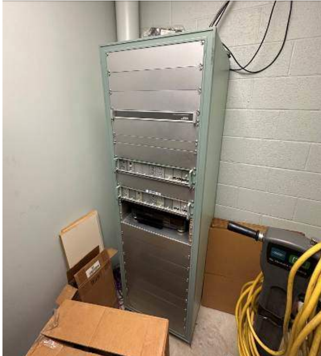
Existing Media Retrieval Rack
