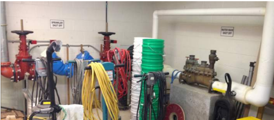
Combination Fire and Water Service and Sprinkler Backflow Preventer
