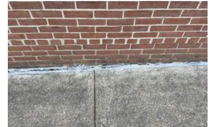
Figure 17 - Eroding Caulk Joint
