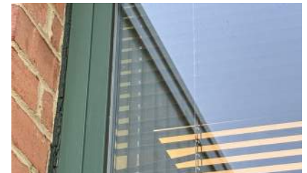
Figure 18 - Eroding Caulk Joint
