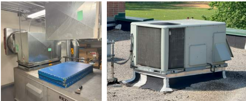
Existing Gymnasium H&V Unit and Gymnasium Lobby Rooftop Unit (Shown Above)
