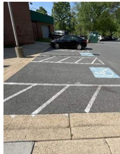
Figure 6 – Non-Compliant ADA Parking Spaces
