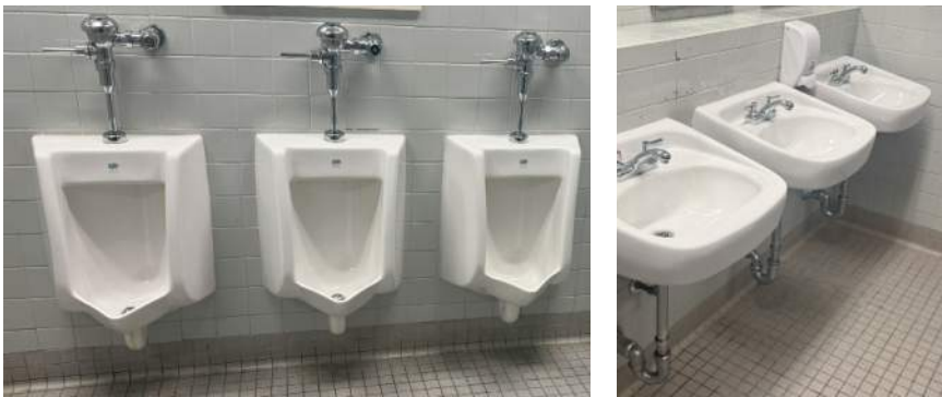
Existing Urinal and Lavatory Plumbing Fixtures
