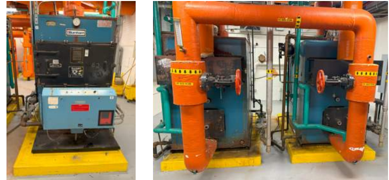
Existing Heating Water Boilers (Shown Above)
