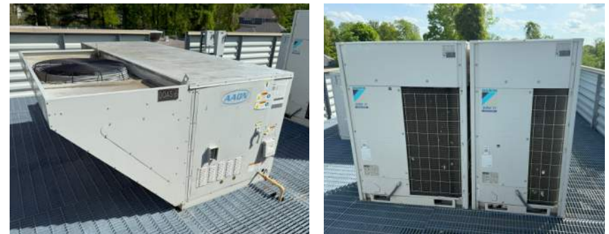
Existing Rooftop DOAS and VRF Air-Cooled Condensing Units (Shown Above)
