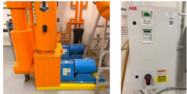
Existing Chilled/Heating Water Pumps and VFD (Shown Above)
