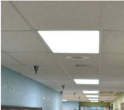
Existing LED Luminaires)
