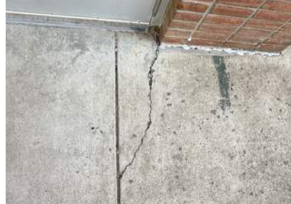
Figure 21 - Crack in Concrete
