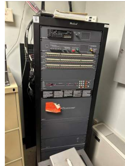
Existing Intercom System
