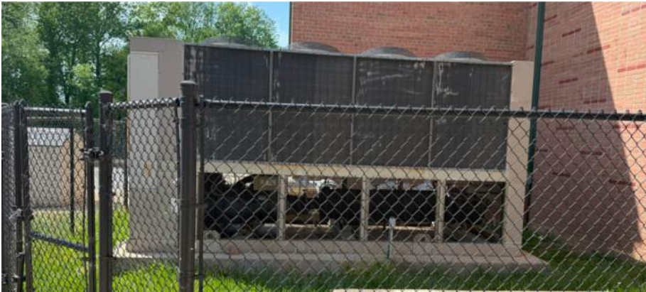
Existing Air-Cooled Chiller (Shown Above)
