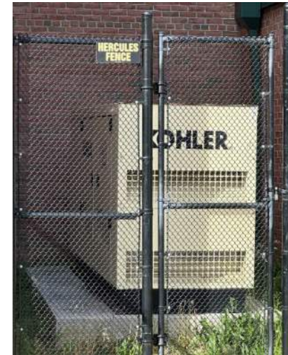
Existing Kohler Emergency Generator
