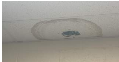
Figure 34 - Ceiling Tile Damage
