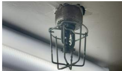
Figure 52 - Rusty Sprinkler Head
