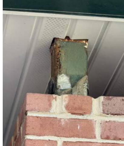
Figure 20 - Rusty Steel Column
