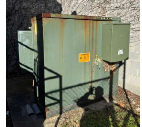
Utility Transformer, Generator, and Cooling Tower
