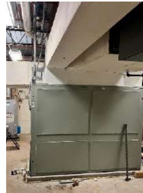
Existing Student Dining Air-Handling Unit
