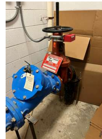
Incoming Fire Service/Backflow Preventer
