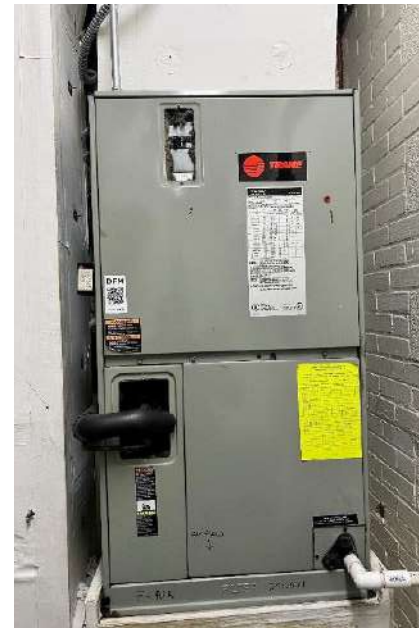
Existing Fan Coil Unit #1
