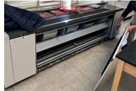
Typical Classroom Unit Ventilator
