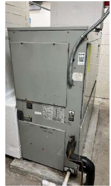
Existing Air-handling unit (AHU-3)
