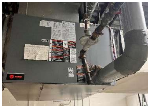
Existing Student Dining Duct Heating Coil
