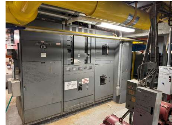
Main Service Switchboard
