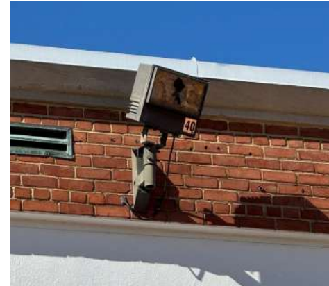
Exterior Wall Pack Lighting Fixture
