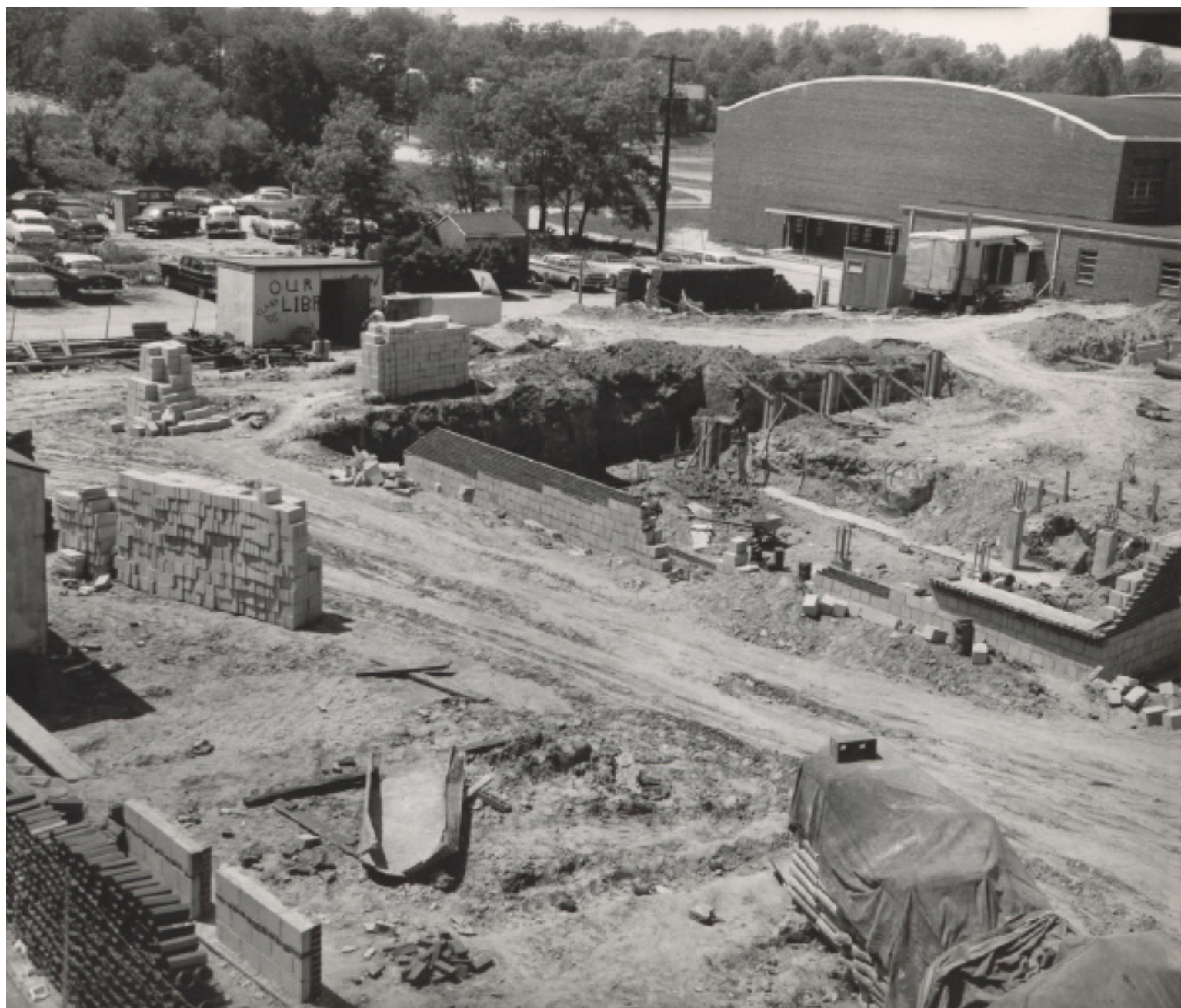
The foundation of the new music building is being laid in the foreground. B-CC has undergone many extensive renovations and expansions since its first years. The most recent one began in 1999, and integrated a traditional facade with a modern interior. Photo courtesy of The Tattler.
