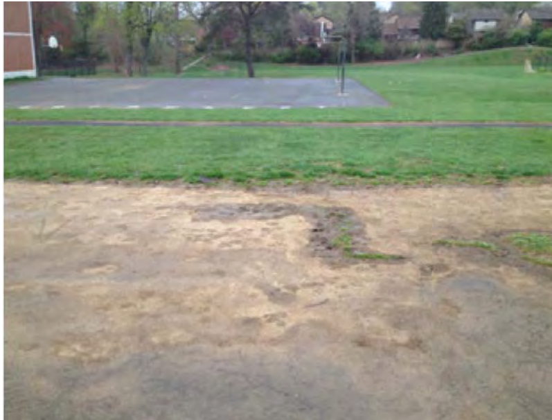
Sediment deposit on hard activity surface
