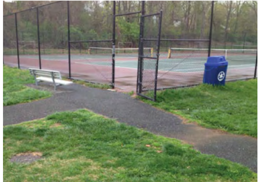
Ponding water on Tennis Courts
