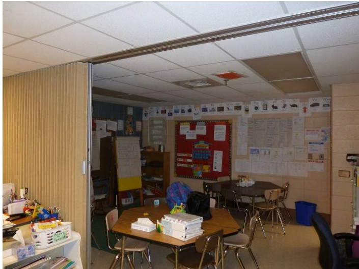
OPERABLE PARTITION AT RESOURCE ROOM
