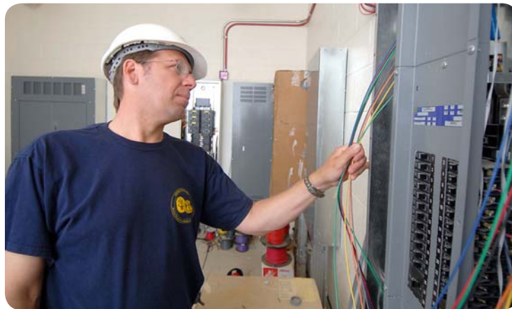
Richard Vanderlinden inspects the electrical wiring at the new Arcola Elementary School under construction. The school is scheduled to open in the fall.
