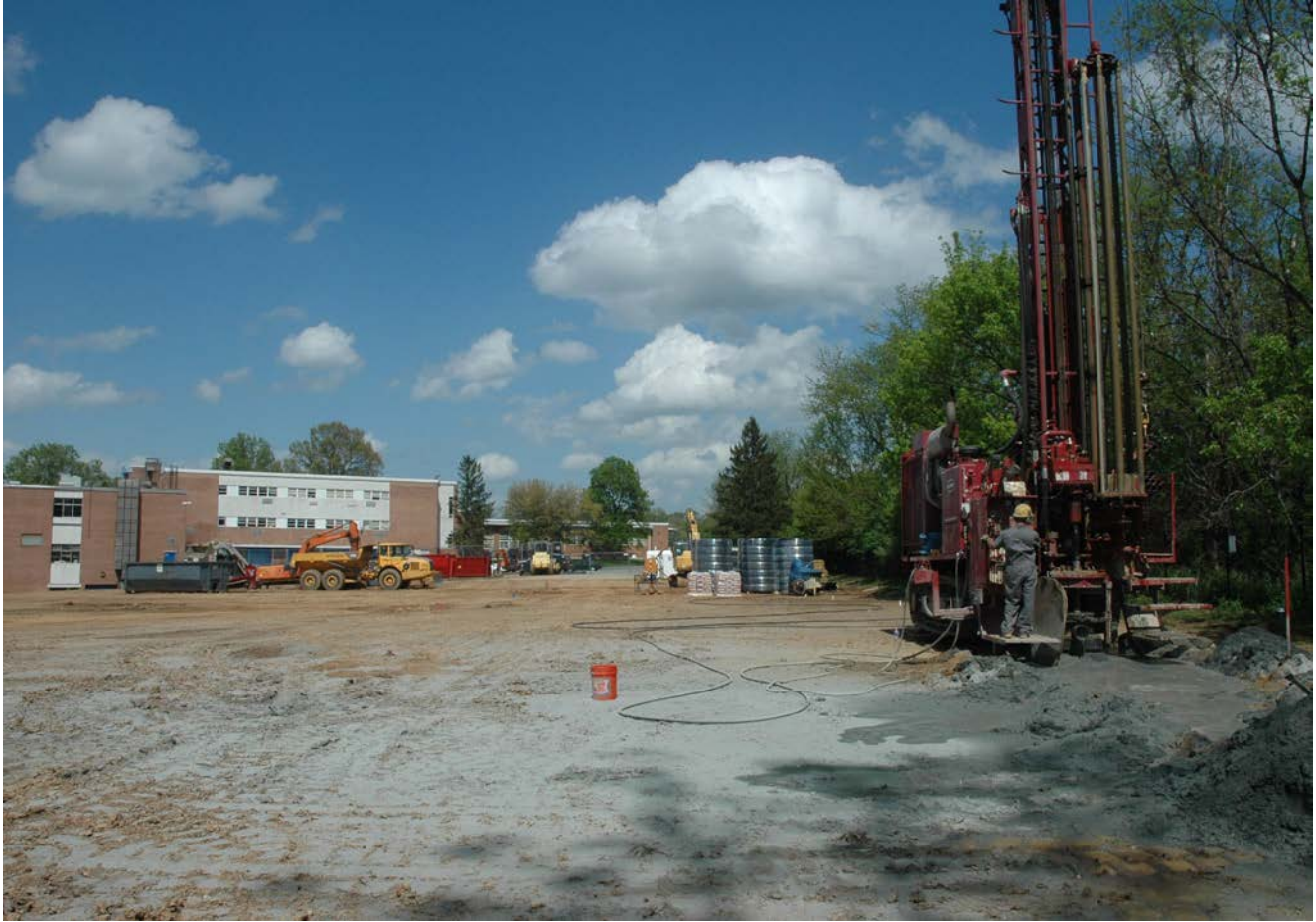
Pictured above: Boreholes being drilled for a geothermal heat pump system at Gaithersburg High School
